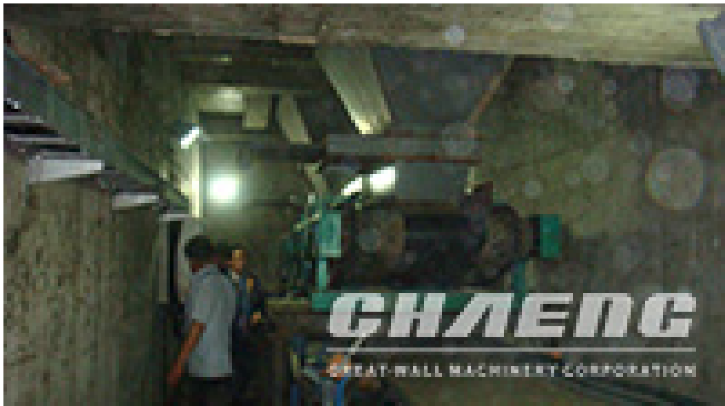
Feeder in 600,000 t/a production line of CHAENG
